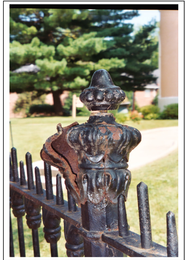
Cast iron is very susceptible to water damage, which can lead to rust and cracking.
