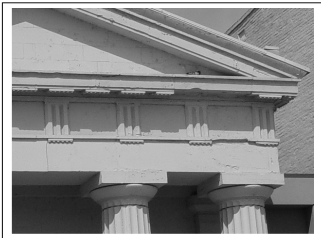
Elements visible on the former Indiana State Bank include pediment (top), cornice (middle) and frieze (bottom)
