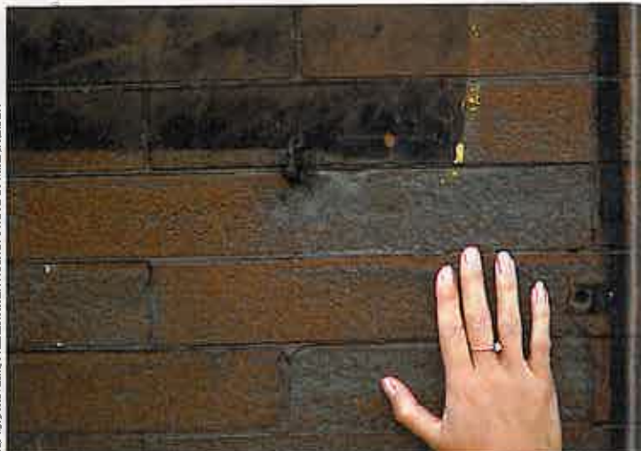
LEFT: Unnecessary exterior waterproofing can result in trapped water that destroys old bricks. ABOVE: This late 19th-century Chicago, Illinois, townhouse shows pitted scars where paint was removed by sandblasting (the smooth bricks above were protected by a shutter).
