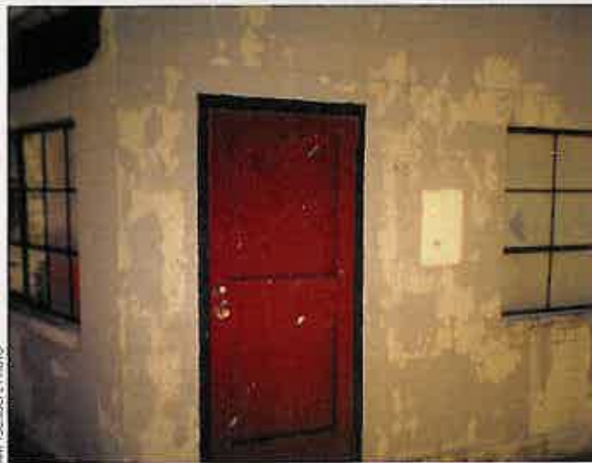
THIS PAGE: A circa 1790 house (top) in the tiny village of Niskayuna, New York, shows a restoration handled properly. Too often, poor prep or cheap paint can result in complete paint failure—like the above example on a building painted just six years ago. OPPOSITE: Repairs gone wrong can result in rot, failures, and cracks.
