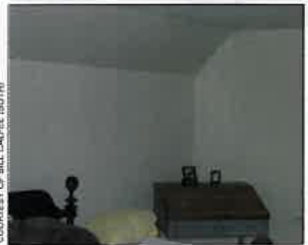
An audit photo shows cold spots where insulation is lacking in an exterior wall—a good place to add fiberglass batts if opportunities for access ever present themselves.
