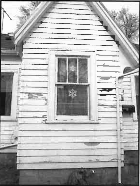
A c. 1936 window that needs to be repaired and not replaced. Photo courtesy of the author
