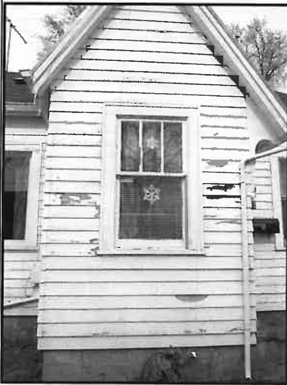
A c. 1936 window that needs to be repaired and not replaced. Photo courtesy of the author
