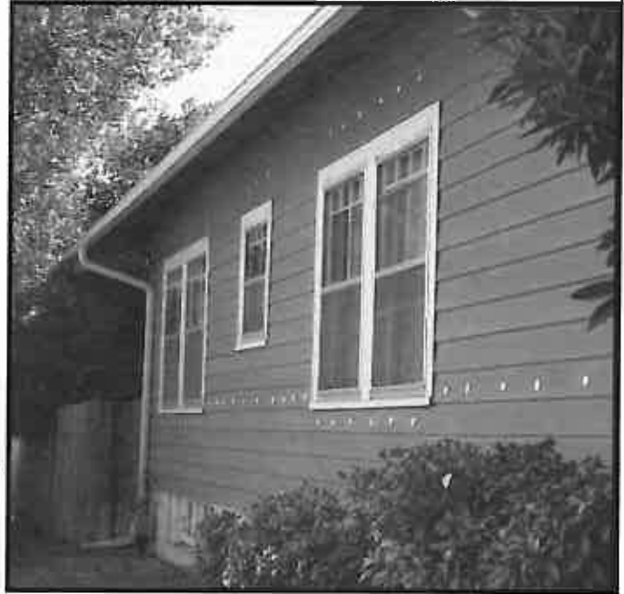
"Woodpeckered" house due to blown-in insulation. Photo courtesy of the author.
